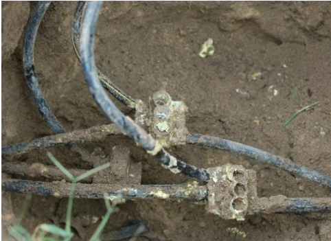
Figure 3: underground pre-meter tap
