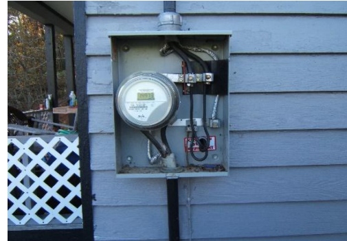
Figure 4: pre-meter tap behind the meter
