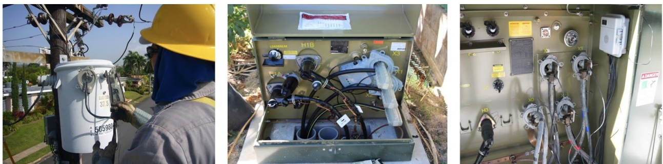
OptaNODE ® DTM and PDTM intra-grid sensors installed on Distribution Transformers
