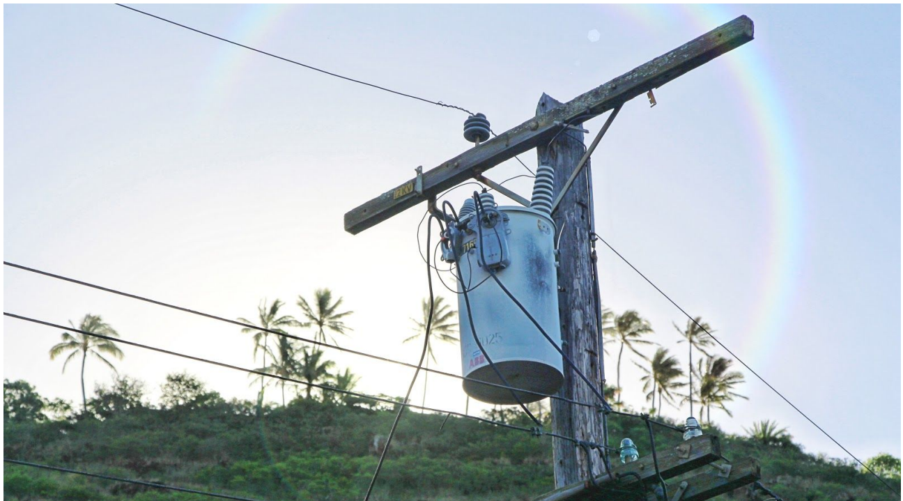
OptaNODE ® DTM sensor installed on overhead Distribution Transformer - Oahu, HI
